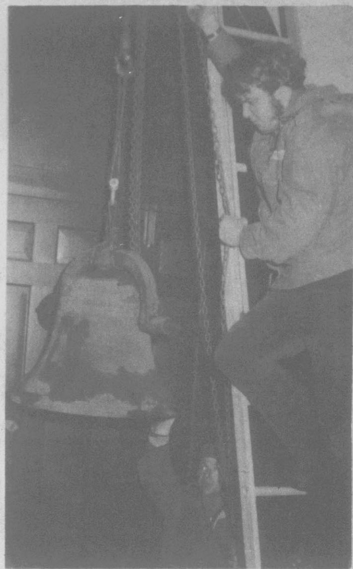
THE BELL COMES DOWN ... but only for a journey to a new home. Above, James Davenport Jr. on the ladder, and Buck Brown, below, help lower the bell from Memorial Baptist Church on Greene St. (Photo by Photo Arts, Greenville)
