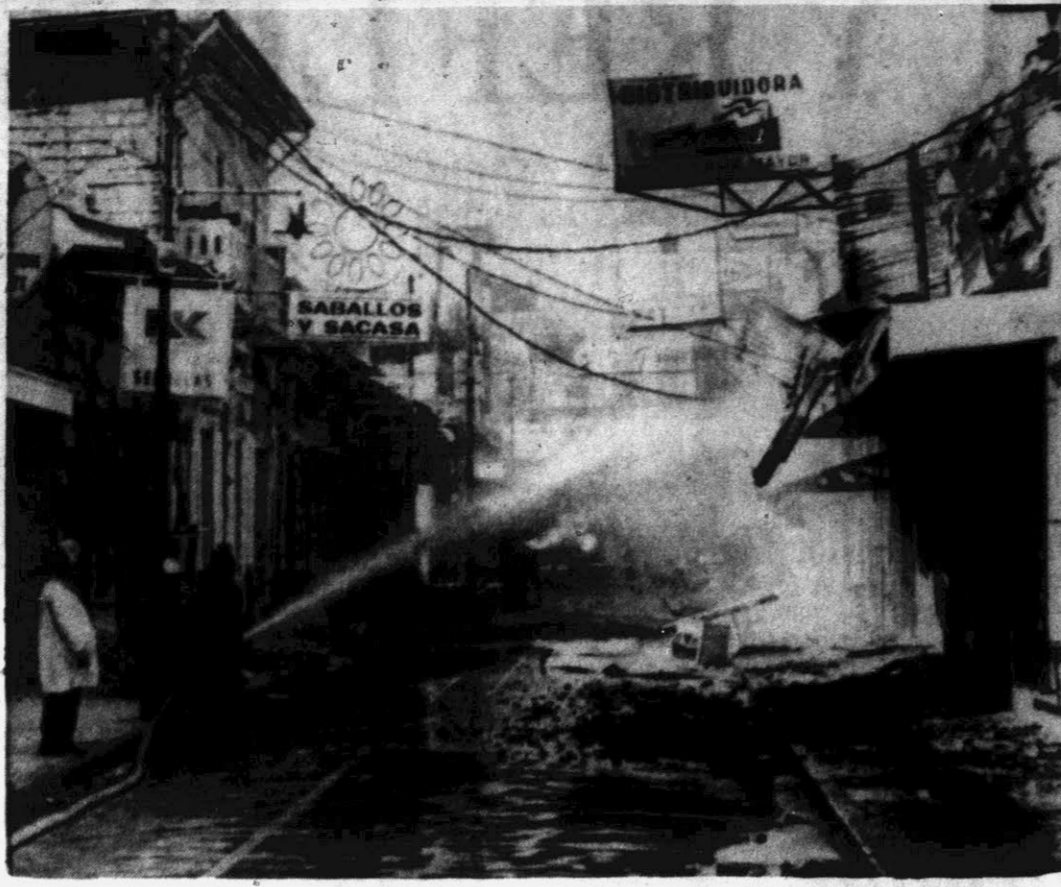
HOISING DOWN THE RUINS — Firemen play water on the smoldering ruins of buildings along a debris-littered street in the capital of Nicaragua, Managua. Demolition crews were still dynamiting and bulldozing in the downtown area Thursday. (AP Wirephoto)
