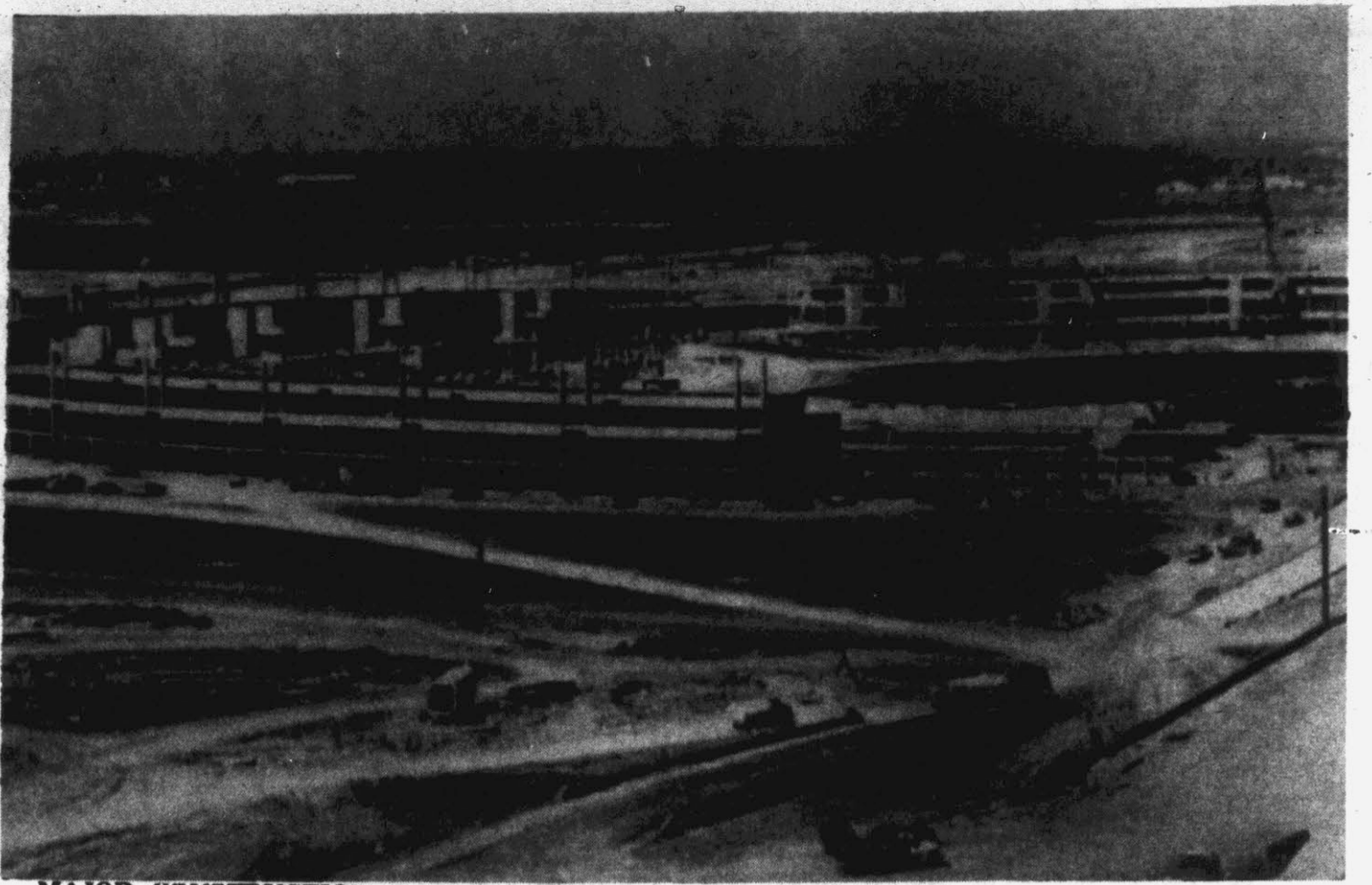
MAJOR CONSTRUCTION work on the Braniff Airport, scheduled to open in the fall of 1974, nears completion. (UPI Telephoto)
