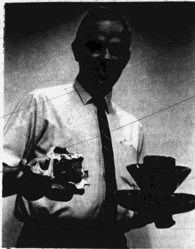
POWER FAILURE . . . Malcolm Green, assistant director of the Greenville Utilities Commission holds broken insulator and new one to compare damage caused by lightning. The insulator held a 34,000 volt transmission line and was blown apart by lightning bolt. (Reflector Staff Writer)
