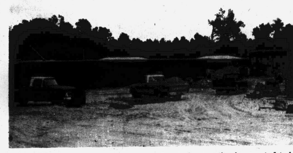
CONSTRUCTION GEAR AND EQUIPMENT... marks the site of the new Wahl-Coates School on East Fifth Street. Construction is expected to be completed possibly by the beginning of November. (Reflector Staff Photo)
