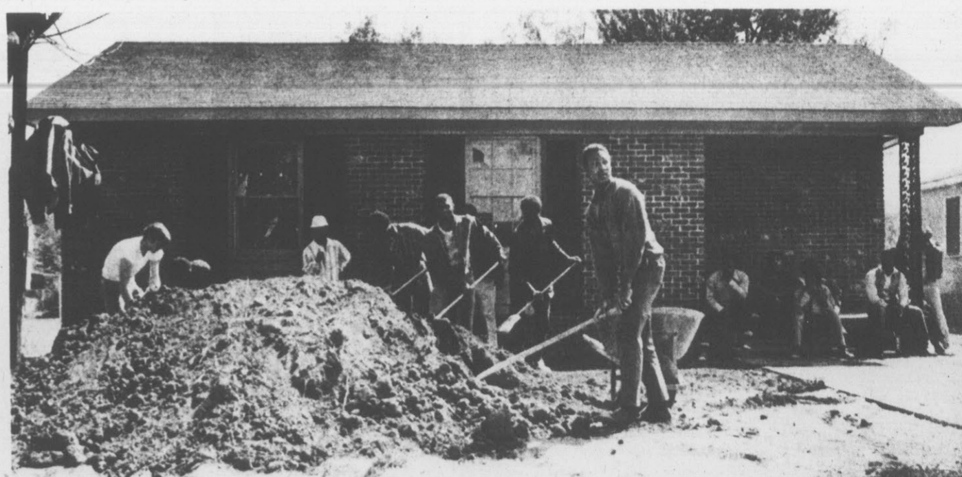
VOCATIONAL EDUCATION . . . students taking turn on the final work of the house they built at 1107
