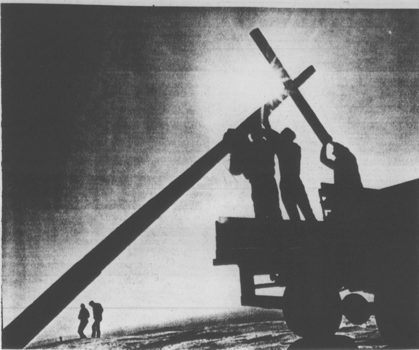
HIGH ON A MOUNTAIN — Workmen raise a cross high atop Stone Mountain near Atlanta, Ga. as they prepare for the sixth annual Sunrise Services Easter morning. A torch lighted walk-up
