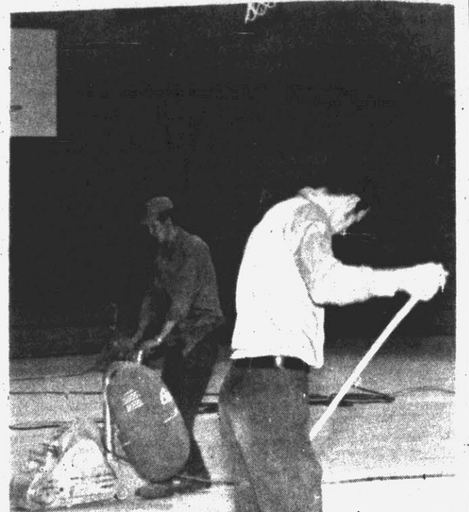
FINISHING TOUCHES . . . Workmen put finishing touches on the gym floor at D. H. Conley High School. Electricians and other workers were also completing their work at the school this week.
