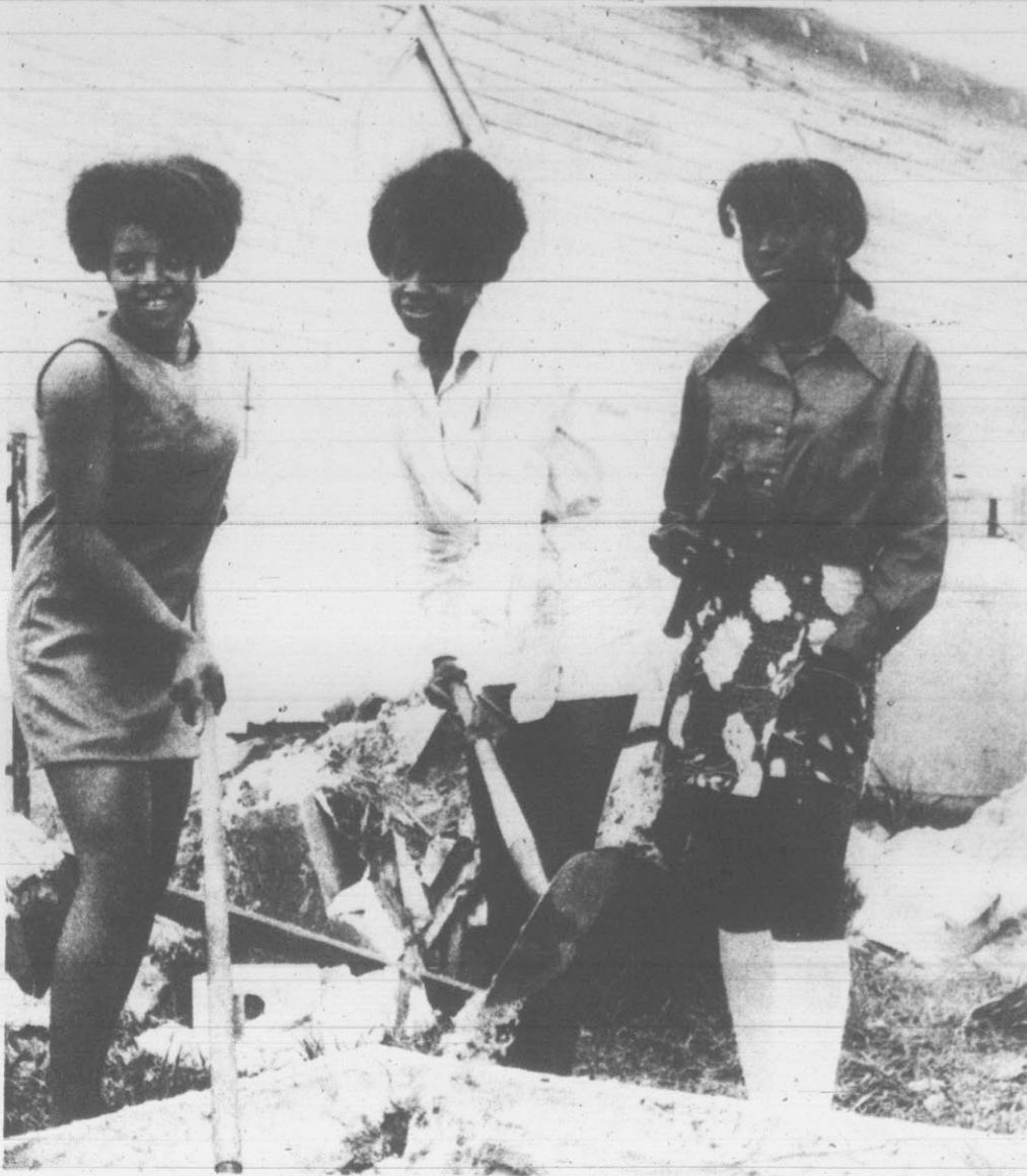
TRIO OF CRUSADERS . . . try their hand at cement mixing. Denise Speight (left), Carolyn Dawson and Virginia Mills, shown above, were three of those on hand last Saturday to lend a help in the Helping Hand Project to restore Allen
