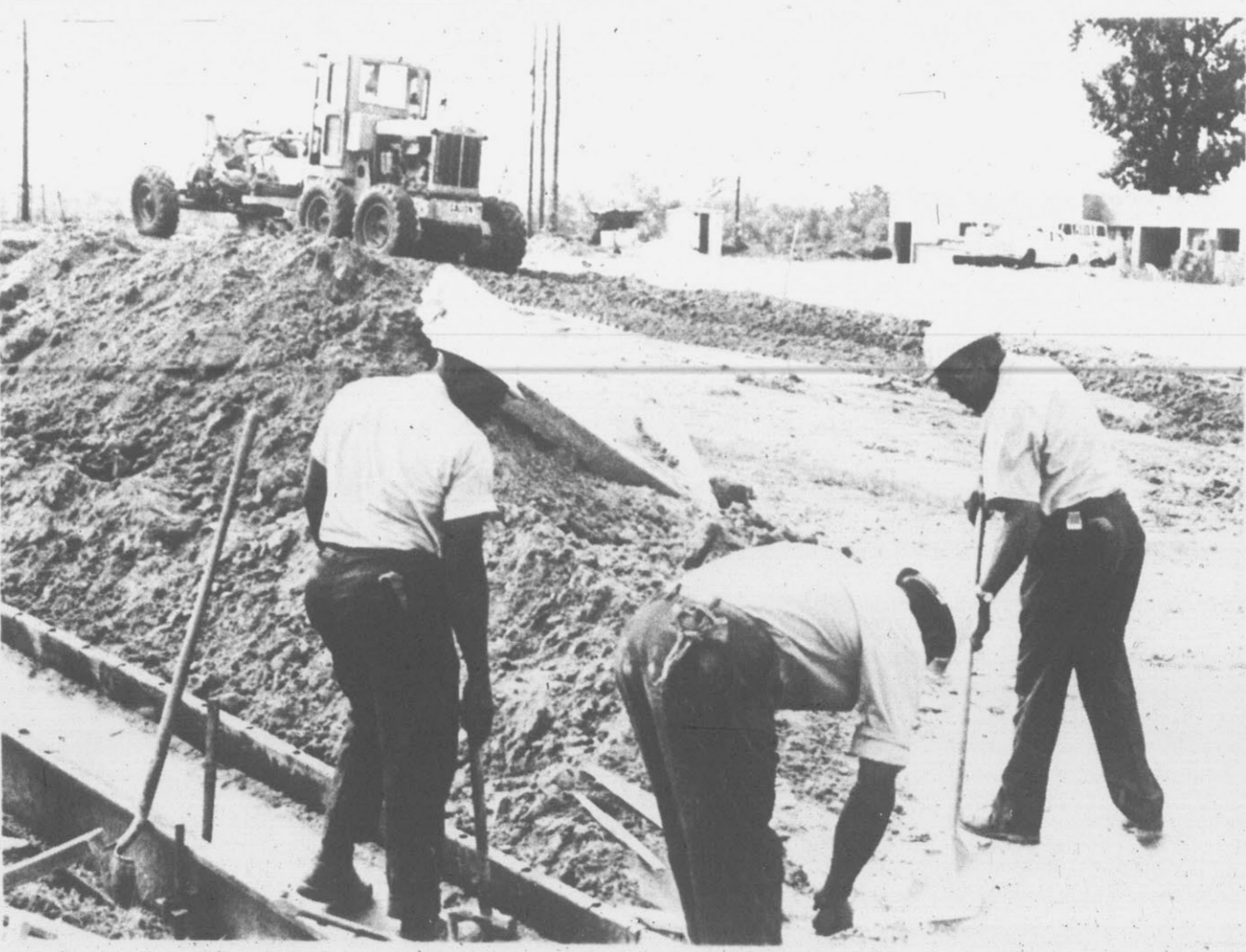
FIRST STREET ... is being extended for a distance of about 200 feet past Pitt Street. City force workmen are shown here aligning curb guides as initial work for the project gets underway this week. (Reflector Photo by Jerry Raynor)
