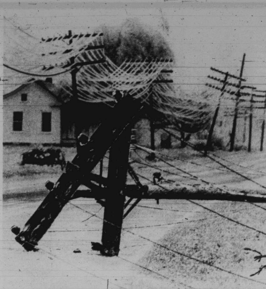
1968 ICE STORM... disrupted power and caused heavy damage in the Greenville-Pitt County area.
