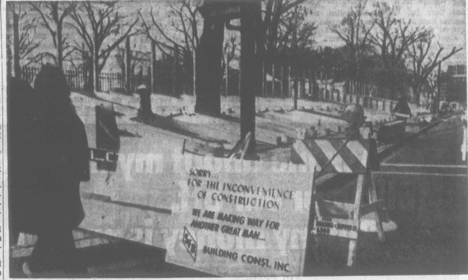
A NEW SIGN ON THE AVENUE — A building firm's sign is in place beside stands being constructed in front of the White House for President-elect Richard Nixon's inaugural parade on January 20. The stands block the Pennsylvania Avenue sidewalk in front of the mansion grounds. (AP Wirephoto)
