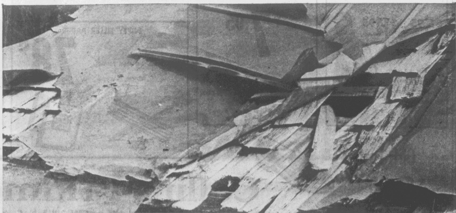
DESTRUCTION OF NATURE . . . wind peeled back the tin roof to reveal wooden shingles underneath.
