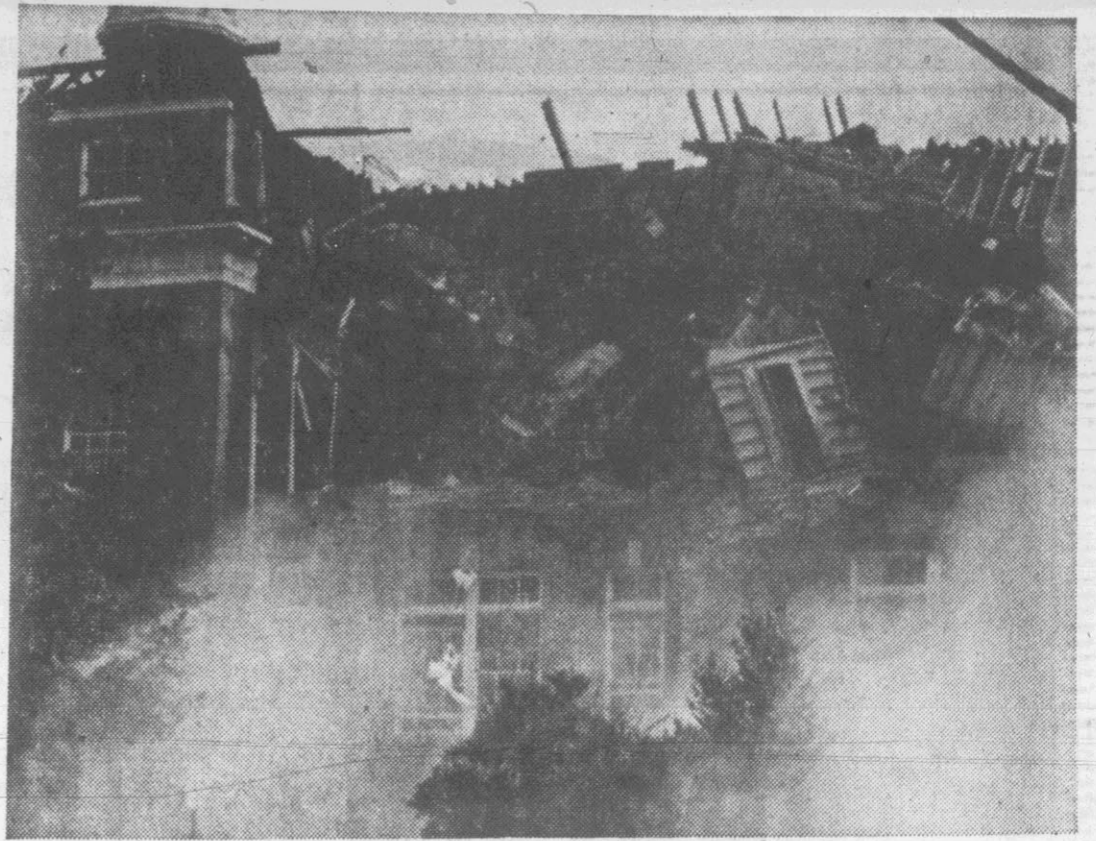
OLD AUSTIN . . . A corner of Old Austin is pulled down by bull dozers yesterday. The collapsing corner sent up a cloud of dust that completely hid the building from view just moments after this picture was taken. (Reflector photo by R. W. Gollobin)
