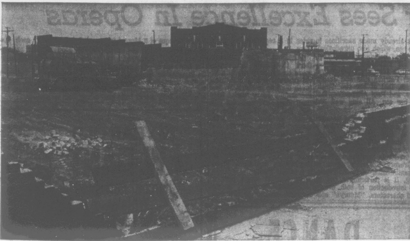
DEMOLISHED CENTRE BRICK WAREHOUSE . . . will be replaced by parking lot for Imperial Tobacco Company employees after gravel and a chain link fence is erected
