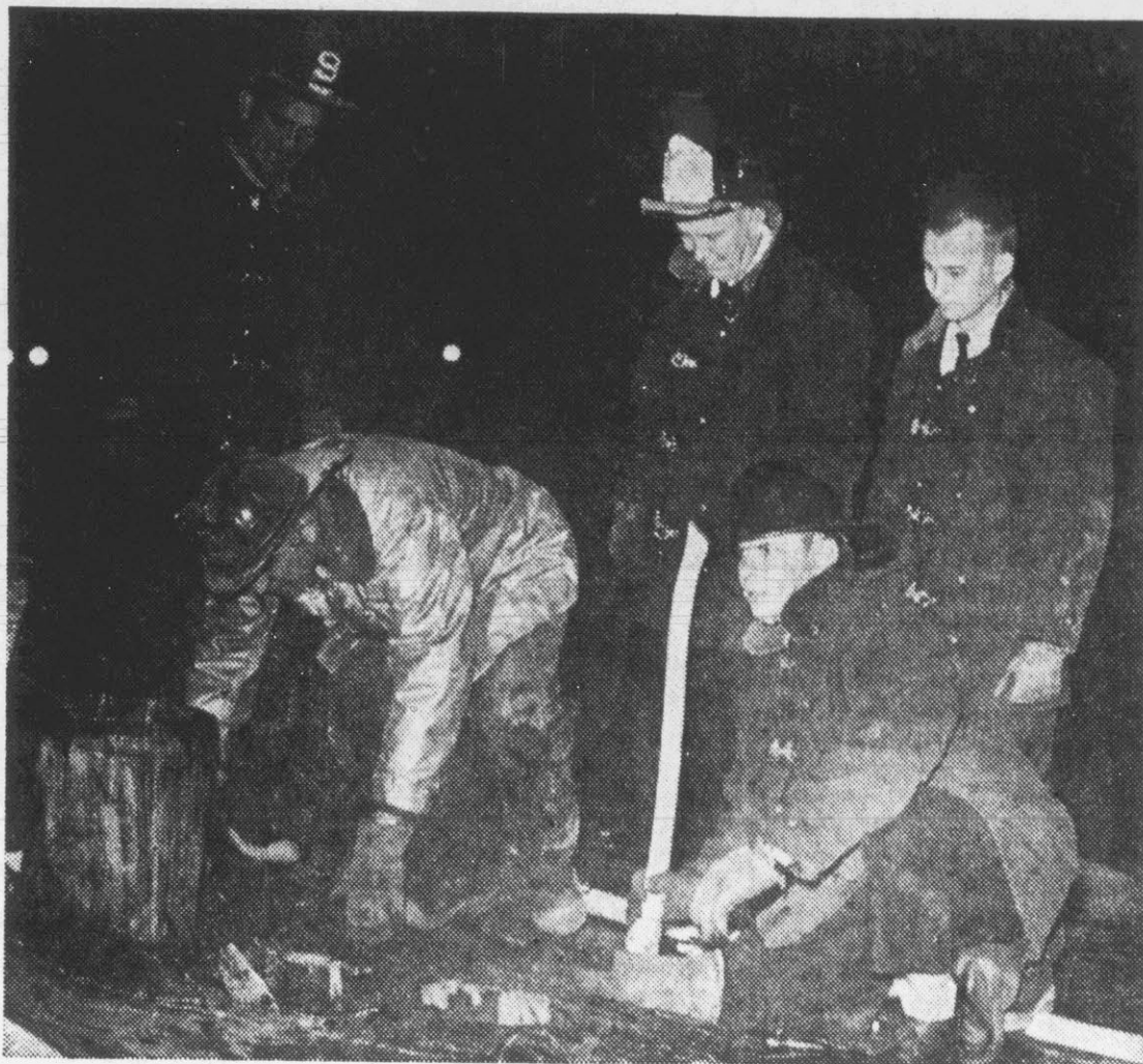
THROUGH THE ROOF... Firemen cut their way through the roof of the Riggs House into the attic where flames had spread from a grease fire Saturday night. (Reflector Photo by Stuart Savage)
