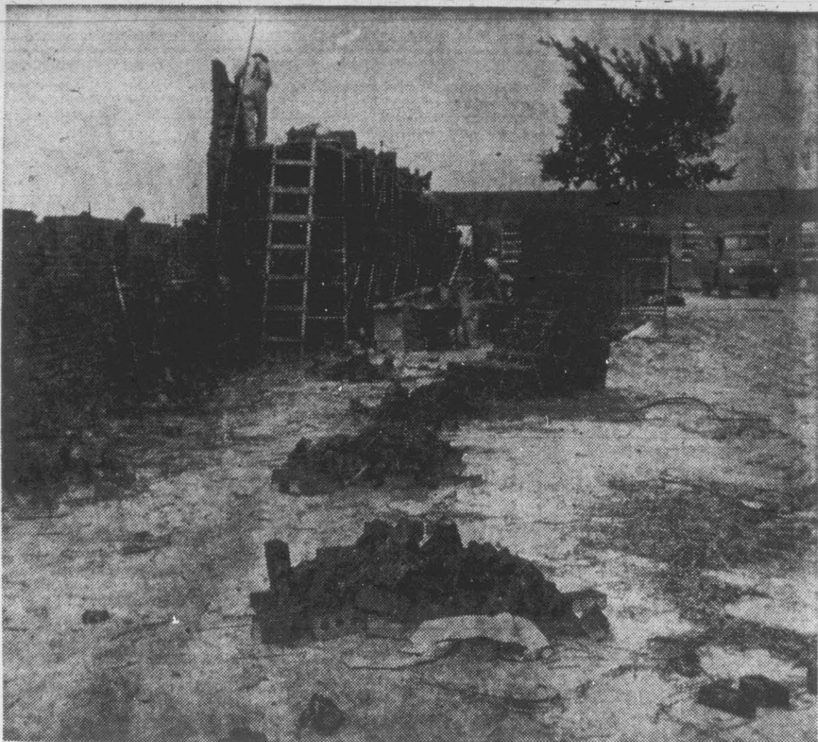
GOING UP . . . Sidewalls for the new Prepshirt Inc. factory are rapidly going up on the North Greenville site, opposite the State Highway Commission shops. Groundbreaking for the plant was held May 24 and construction was started the following week. The 52,000 square foot building is located on a 15 acre site and eventually is expected to employ about 500 people.
