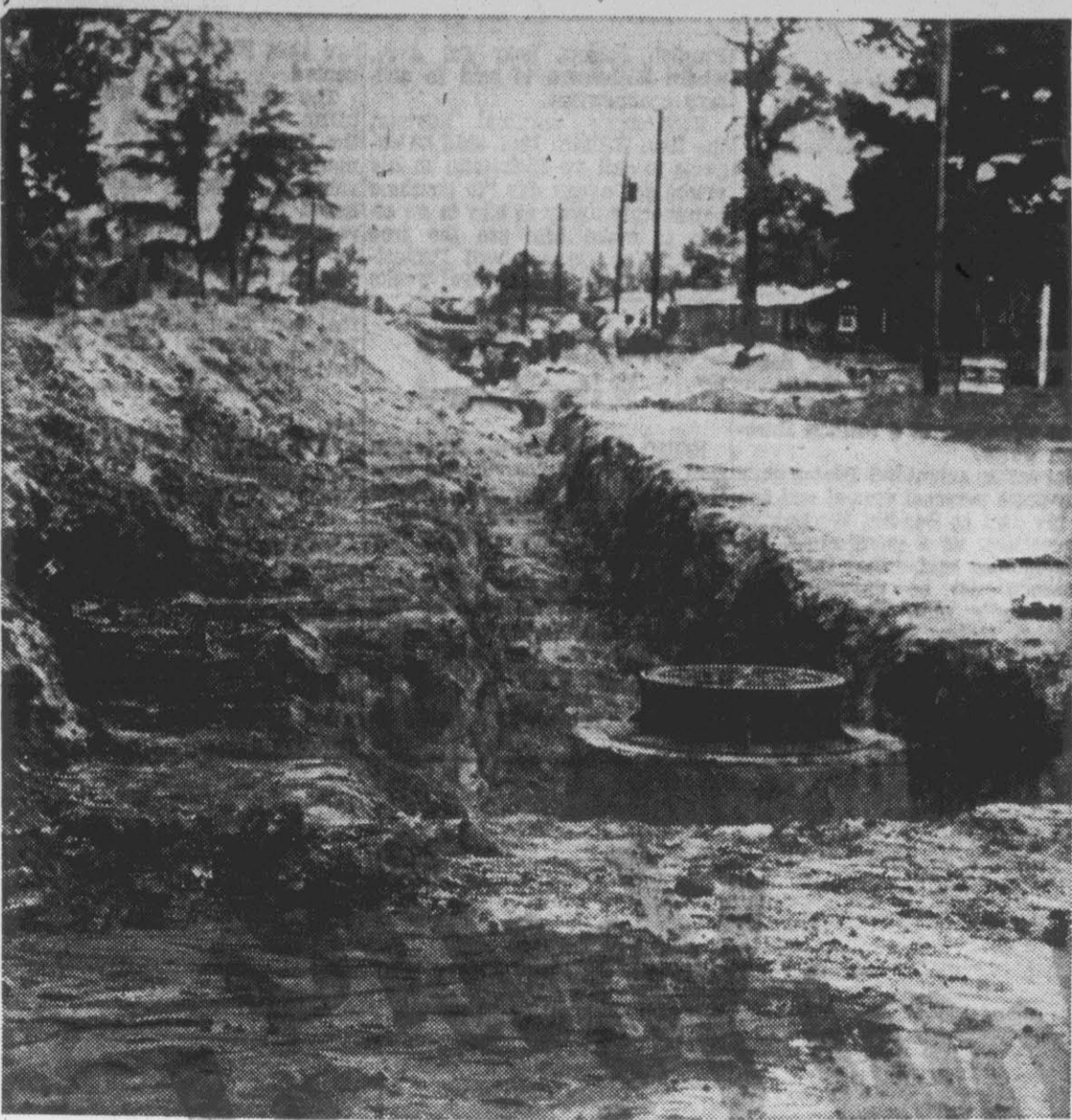
WORK IS IN PROGRESS . . . in Grifton on extension of water and sewer lines. Above, workmen are concentrating on St. Joseph's Street. The work is the result of a bond issue approved last year, to extend water and sewer lines, secure a new well and sewage treatment plant. (Reflector staff photo)
