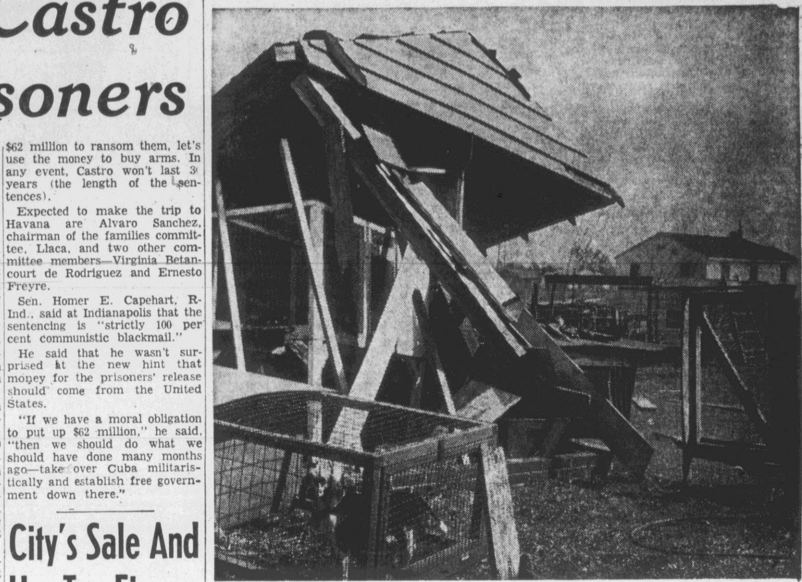
THIS OUTBUILDING . . . a victim of yesterday's storm, collapsed just after owner E. C. Smith ran for his house after seeing the front of the structure come a foot off its foundation. (Reflector, Photos by Stuart Savage. See other photos page 7)
