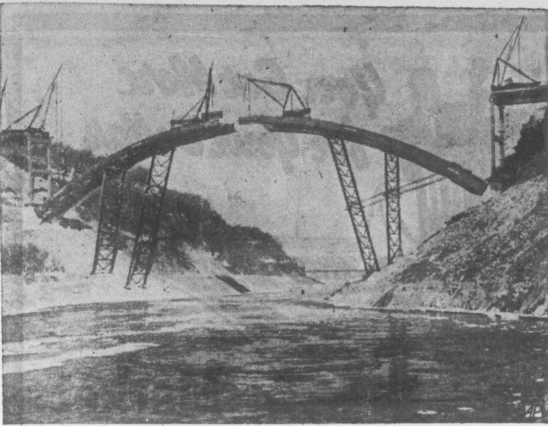
OVER THE BOUNDARY — This is the new bridge linking the U.S. and Canada over the lower Niagara river north of Niagara Falls. The international span will have connecting links to New York State Thruway and Queen Elizabeth Highway in Canada.
