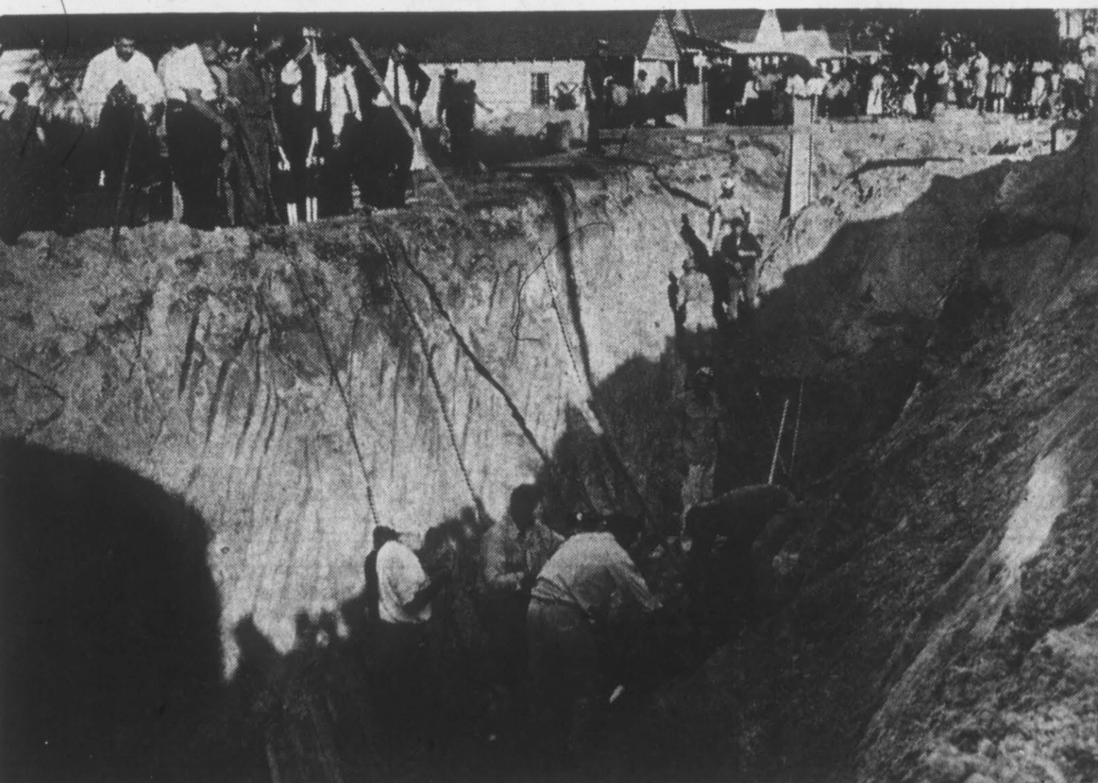
CAVE-IN TOOK THREE LIVES . . . ditch bank gave way as workmen installed sewage interceptor line on West Third St.
