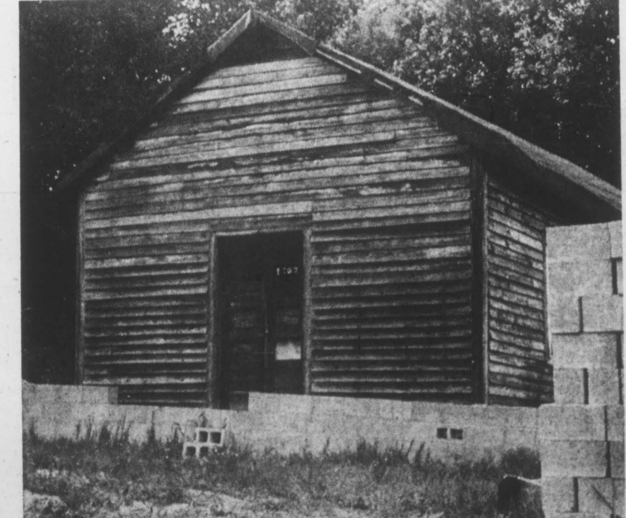
FRONT FOUNDATION . . . for the new Cotton Chapel FWB Church has been laid by members of the church. Work on the remainder of the building will continue next week.
