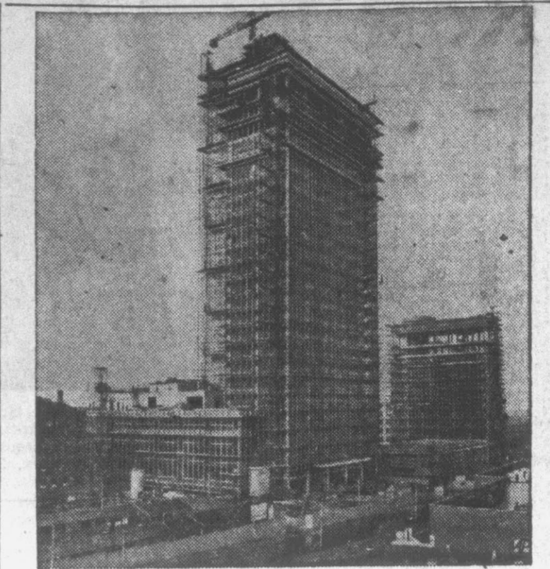
HIGH POINT —The steelwork of Britain's tallest building towers over its Manchester surroundings. The 400-foot high structure will house an insurance company.
