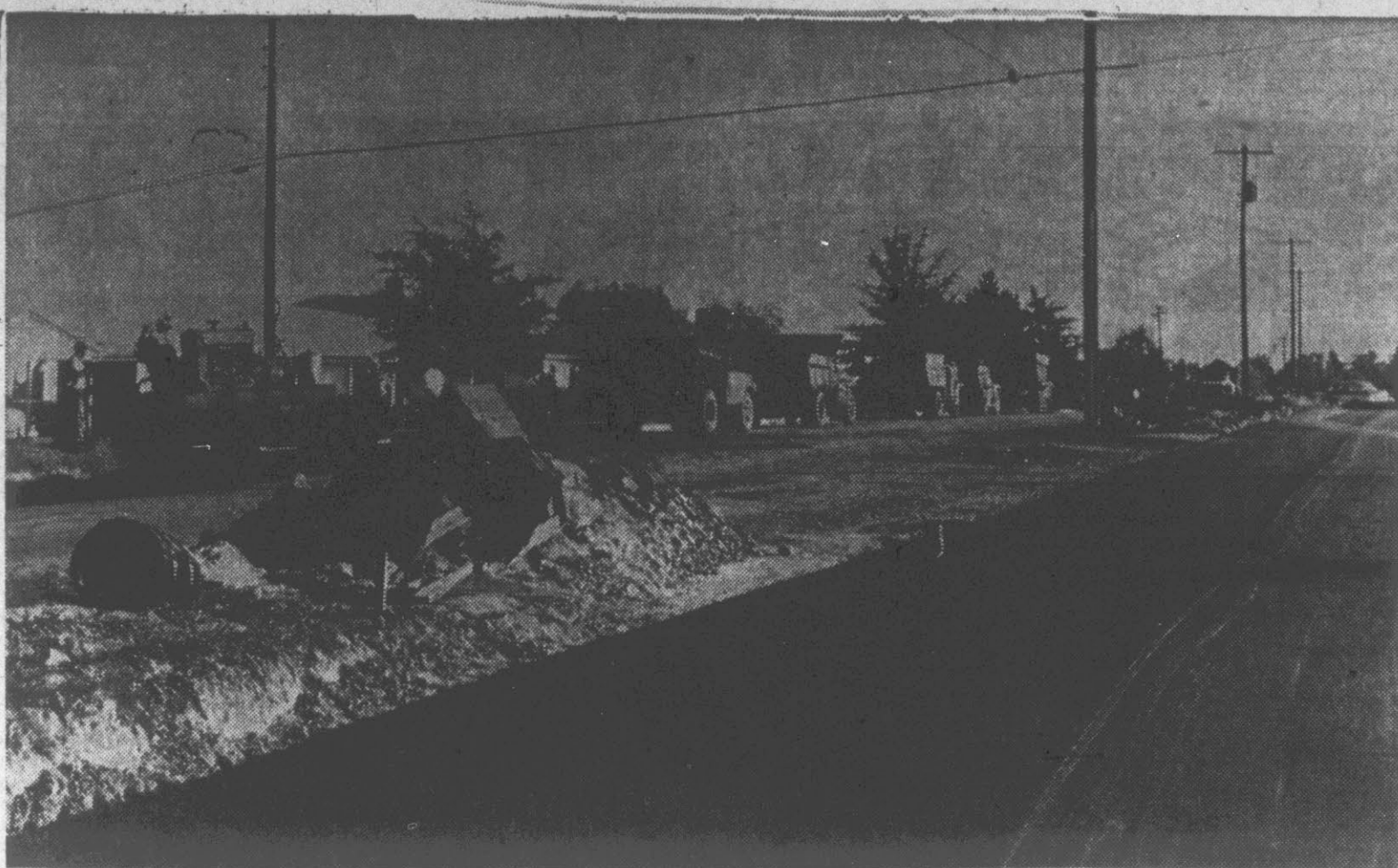
PAVING ON ELM ST.—Paving of the four lanes on Elm St. from Greenville Blvd to Tenth St. was completed Saturday afternoon. Workmen will now turn to the job of installing asphalt curbing around the center islands. City crews will plant grass in the dirt island and shrubbery is to be placed at strategic points. (Reflector Staff Photo)
