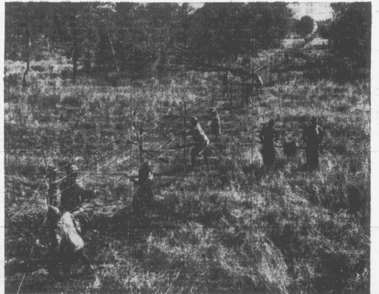
Deep in the bush, workmen erect fence which will completely encircle Kruger Park. When finished, fence will cover distance of 600 miles, making it world's longest.
