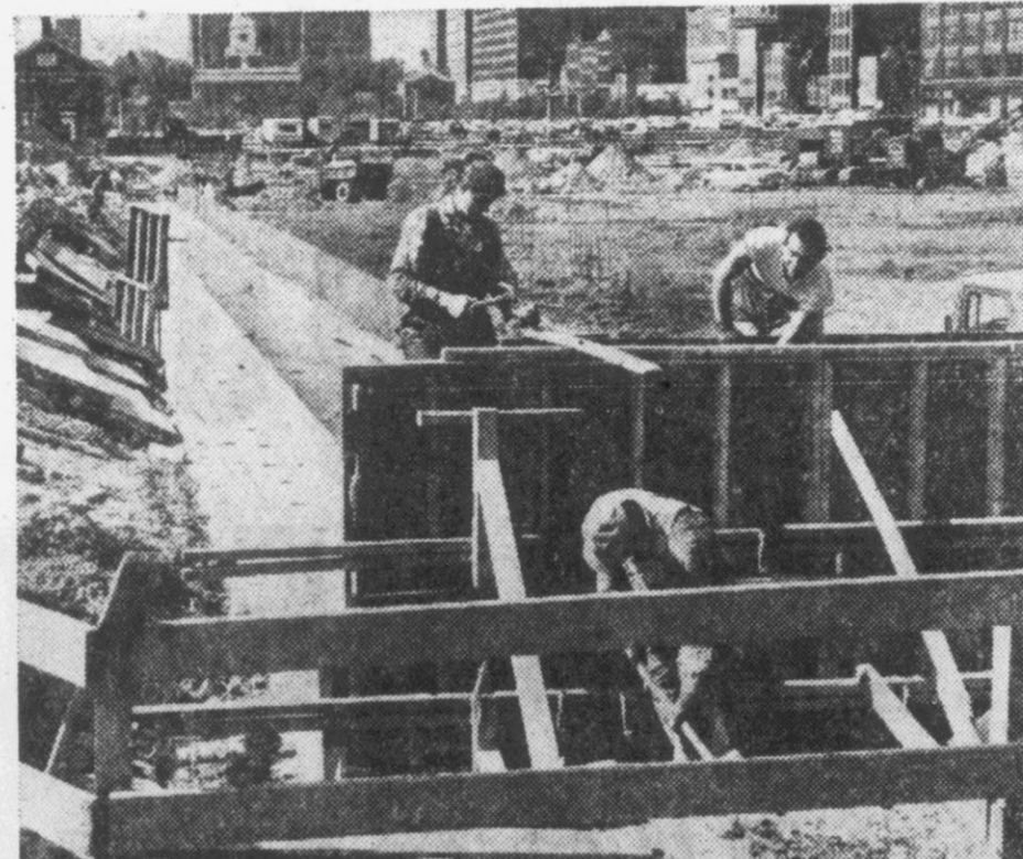
Workmen build retaining wall at northern end of Independence Mall. Many small buildings have been torn down to make room for Mall at far end of which stands Independence Hall. Mall will be landscaped with gardens, walks and fountains.
