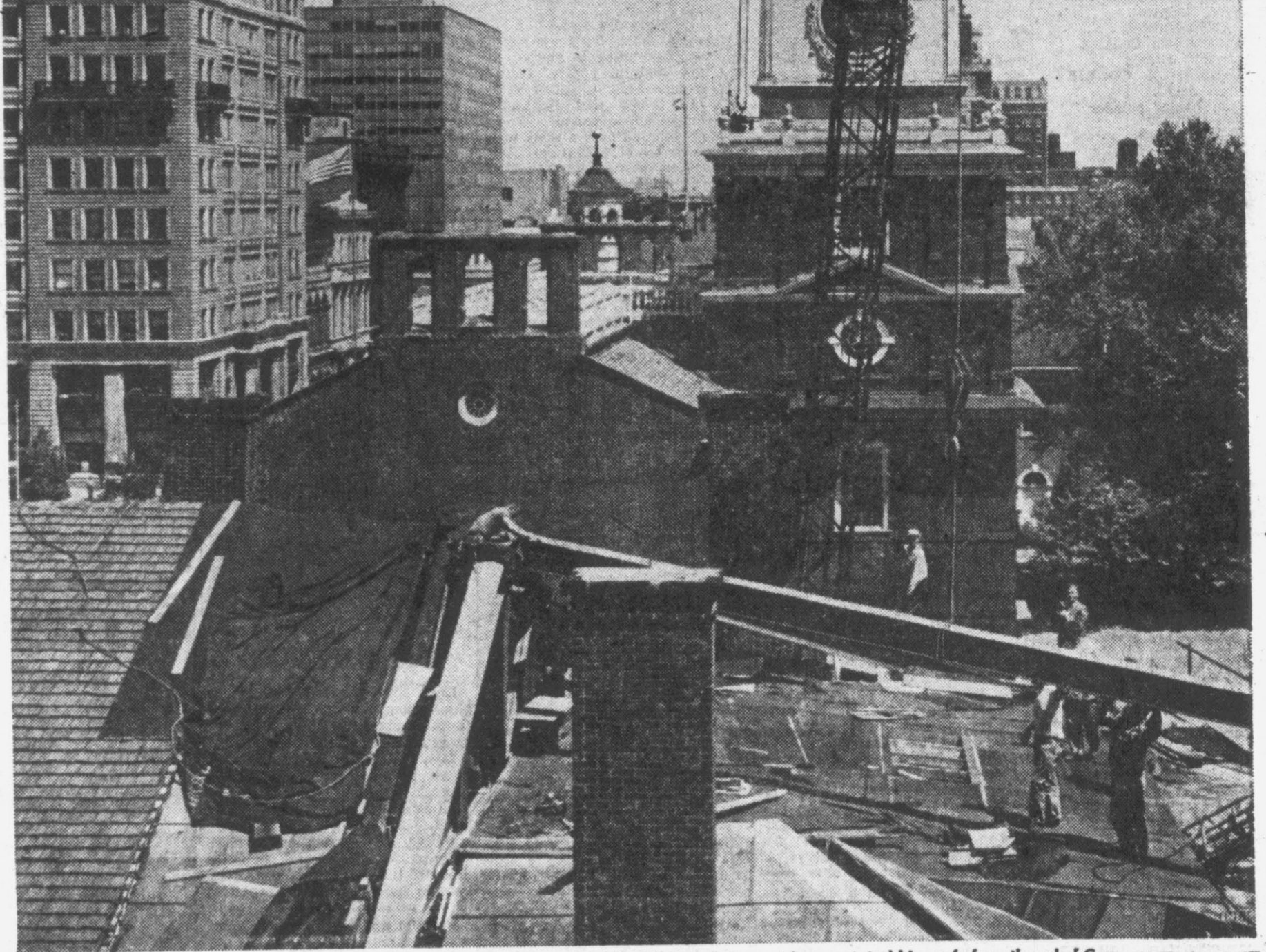
RENOVATING A SHRINE. Workmen swing into place one of steel beams being put in renovated hip-roof of south end of Congress Hall where nation's highest legislative body functioned until 1800. Independence Hall, in background, towers over scene.
