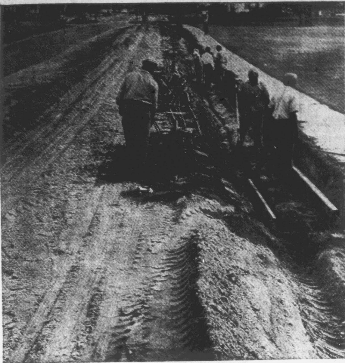
WORK ON ELM . . . Workmen are shown preparing forms for curb and gutter installations in front of Rose High School on Elm Street, in conjunction with the four-laning of the busy street. A four-lane bridge over the Green Mill Run, and part of the project, was completed a short time ago. The widening of the street is being carried out with money appropriated in the recent bond election.
