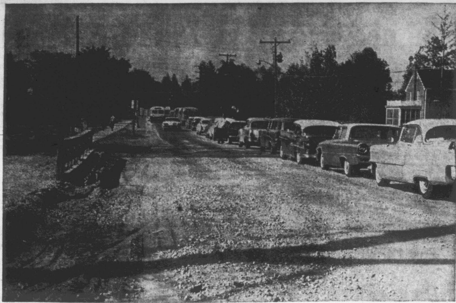
CULVERT IS INSTALLED—Traffic is moving across Greene Mill Run on Elm St. again after installation of a four lane culvert under the street. The work was done by city crews in preparation for construction of a four-lane drive from Tenth St. to Greenville Blvd. The work is a part of the city's street improvement program currently being carried out with bond issue funds. (Reflector Staff Photo)
