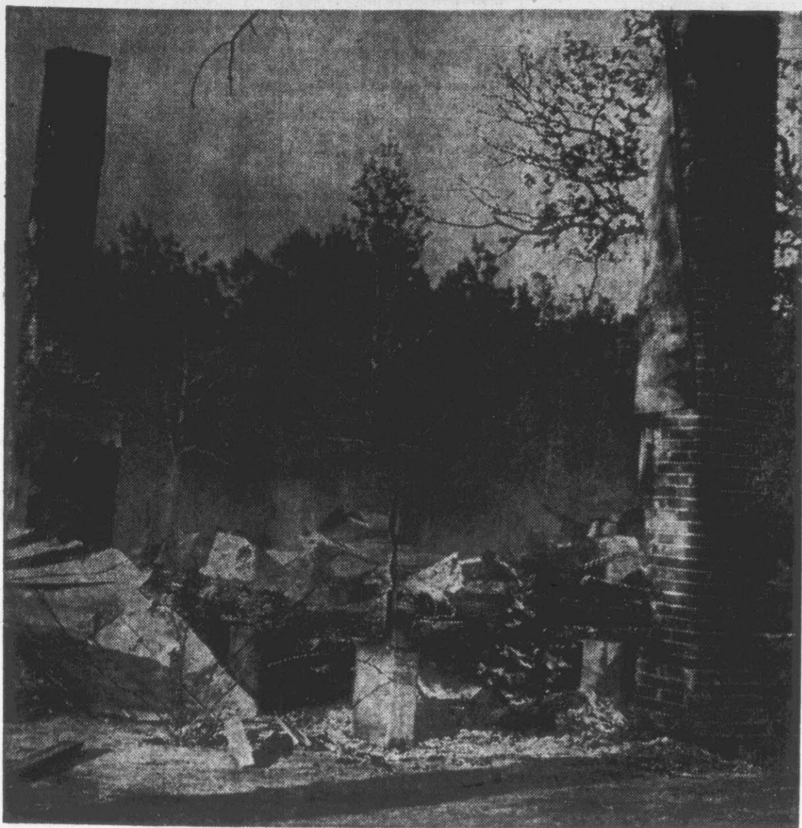
DESTROYED BY FIRE... yesterday was this six-room house on the Galloway farm about two miles west of Grimesland. The house, owned by Mrs. W. S. Galloway of Greenville, was occupied by the Raymond Williams family. Officials of the Grimesland Fire Department, which responded to the call, said the blaze was discovered between 4:00 and 4:30 p.m. when members of the family, working in a field nearby, saw flames coming from the roof of the dwelling. According to Mrs. Galloway, the house was insured, but the Williams family's possessions, of which only little was saved, were not. An electrical shortage is thought to have been the cause of the blaze.
