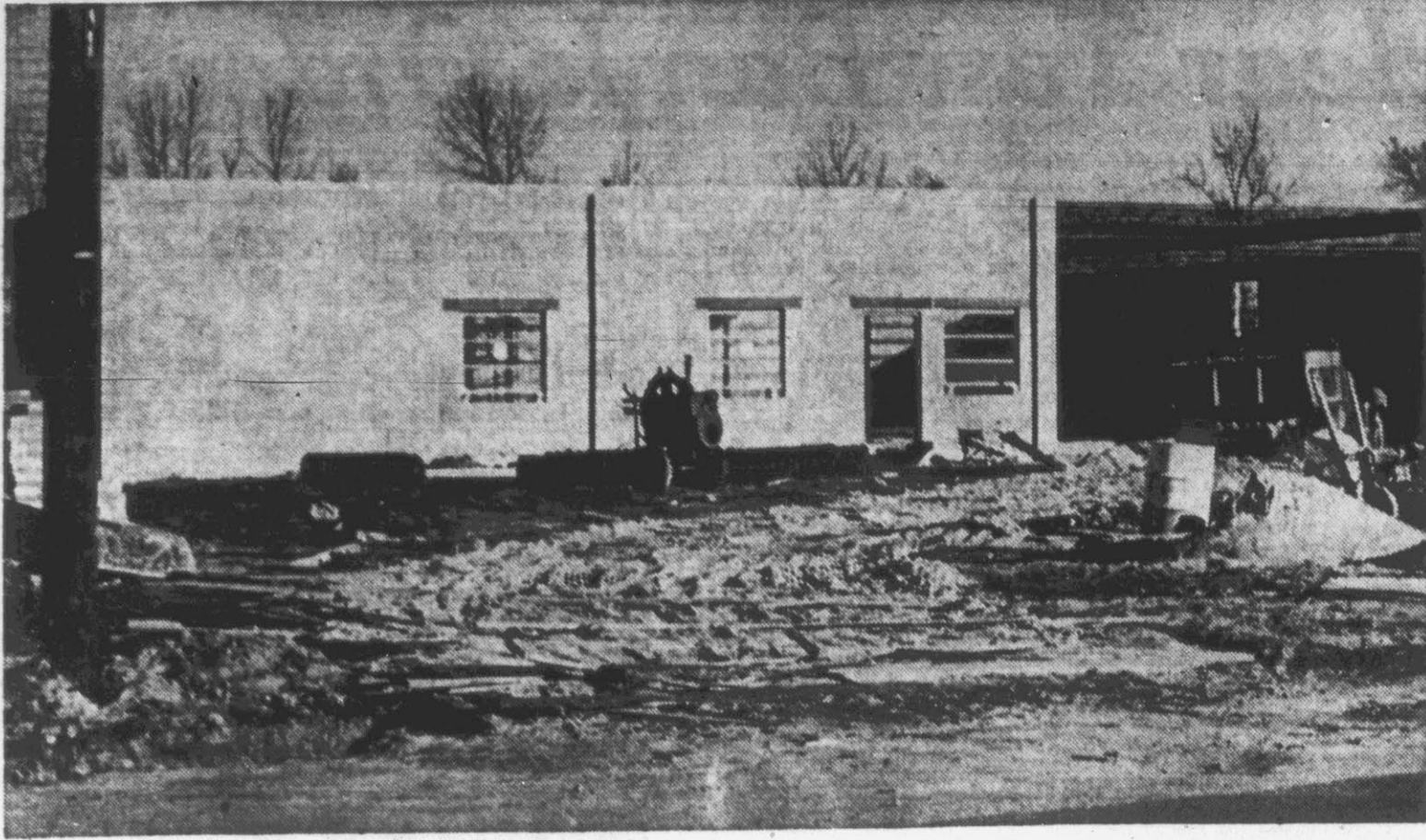
WELL UNDERWAY—This 10,000 square-foot plant, the new home of Farmville's North State Garment Co., is being completed according to a schedule that calls for occupancy by the garment-producing company early in April. Plant manager Thomas Anderson said today he plans to move his operation into the new quarters "between April 1 and 15." The masonry and steel structure will eventually allow Anderson's operation to expand from 64 employees to around 90. Financed by W. A. Allen of Farmville, the building will be leased "to the garment industry. It is located on the east side of S. Main St. in Farmville near Marlboro.
