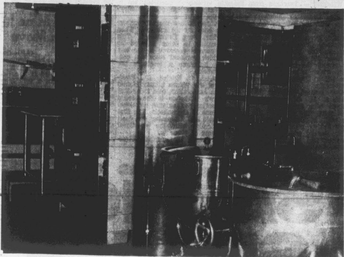
LARGER KITCHEN FACILITIES . . . will be available now. The large kettles and an oven, used in feeding large numbers, are visible here.
