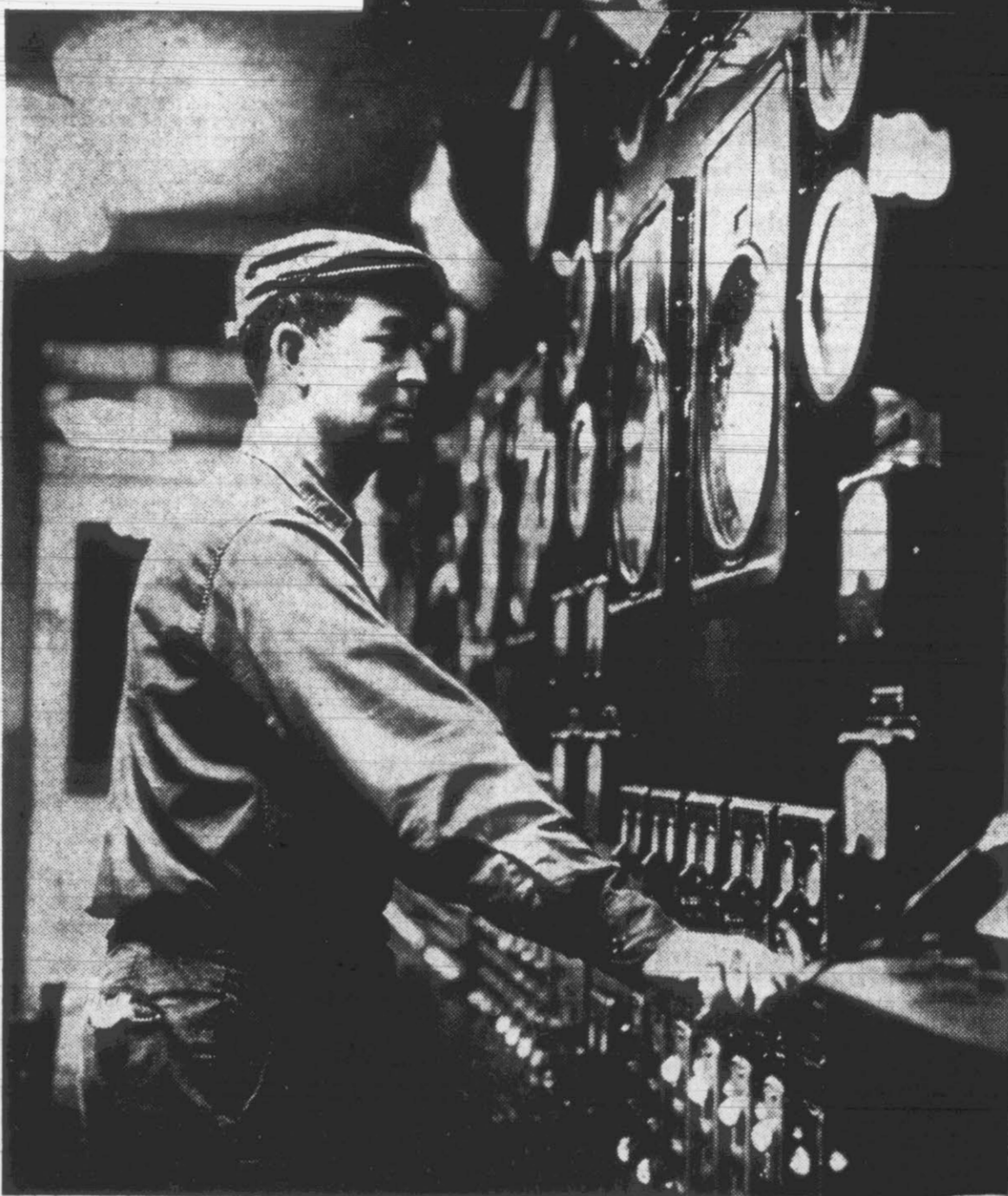
CONTROL ROOM NEAR BOILERS . . . which contains combustion control panel.
