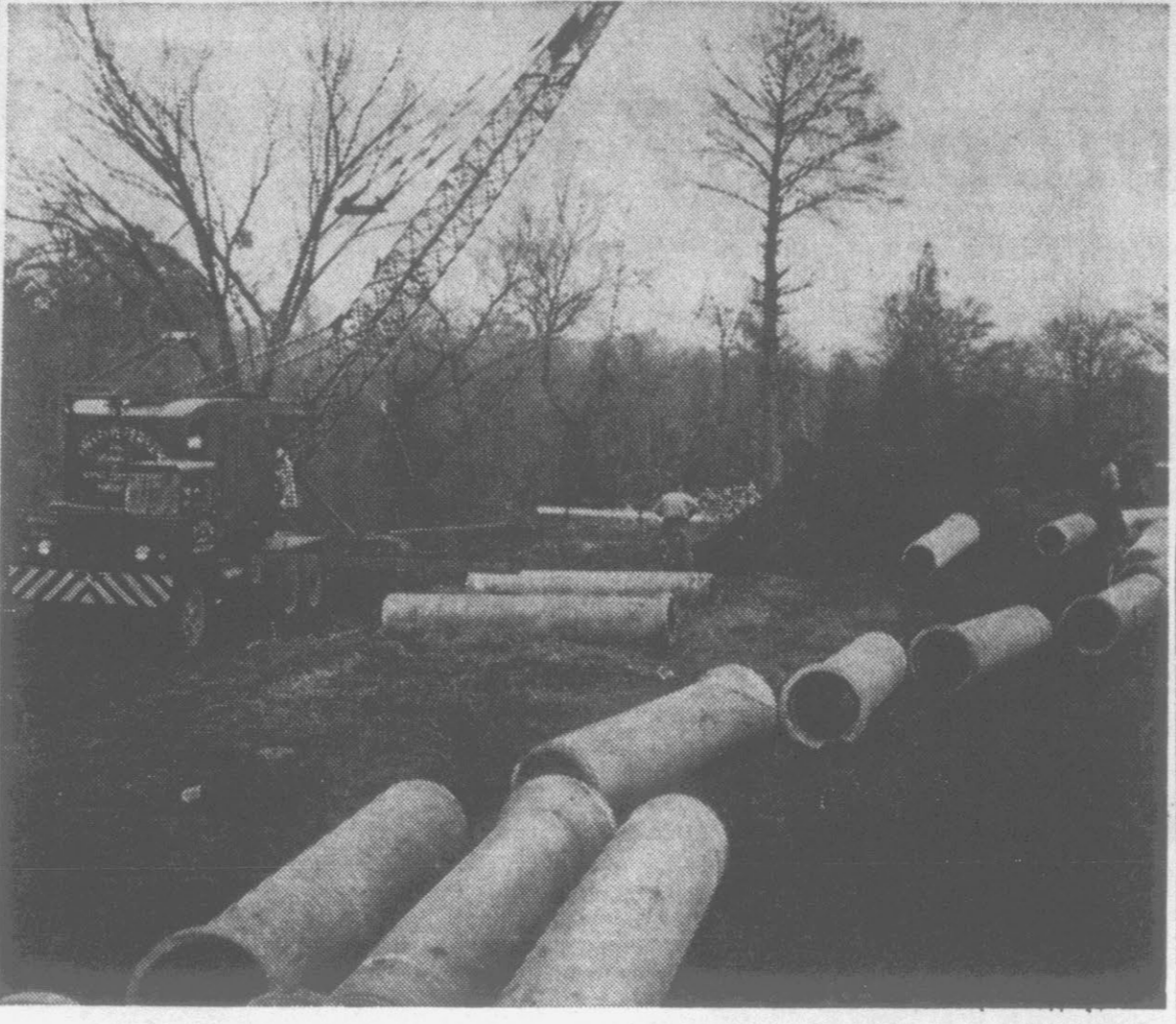
SEWER LINE PROGRESSES—A big crane has been evident at the foot of Evans and Washington Sts. on the river bank this week. It is at work on the sewer outfall line which will serve the city's sewage disposal plant, now under construction behind Greenwood Cemetery. The line will run from Memorial Drive to the plant site, the complete length of the city. (Reflector Staff Photo)
