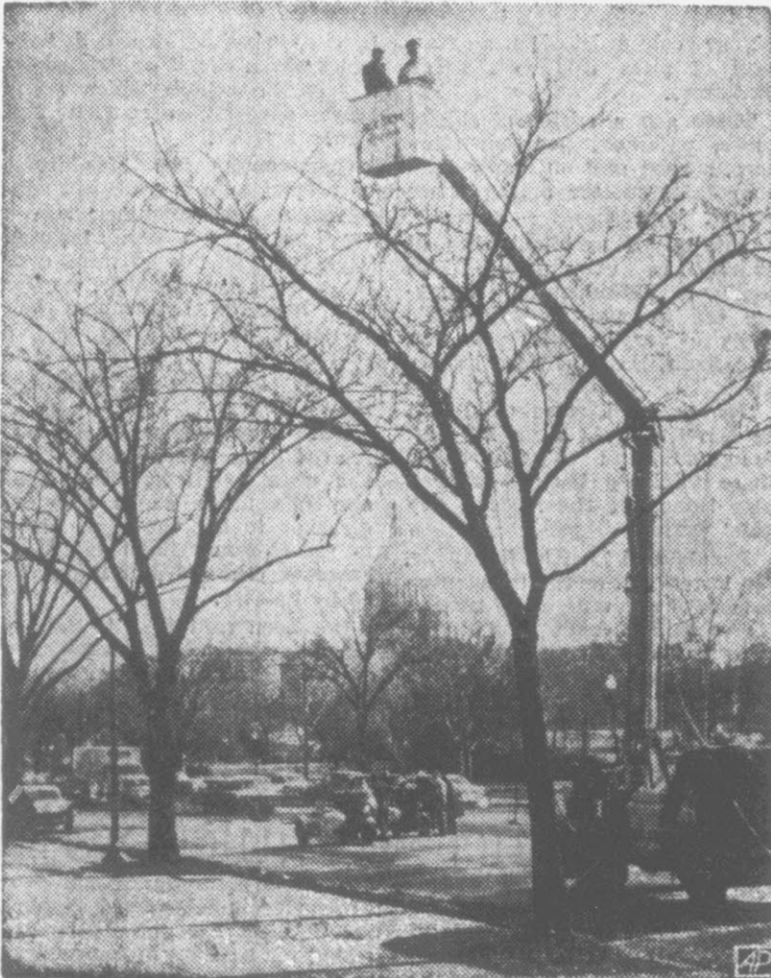
IT'S FOR THE BIRDS—Using a special crane boom, workmen begin bird-proofing trees along the inaugural parade route in Washington. Workmen in the box-like stand at top of the boom are spraying trees along Pennsylvania Avenue with a liquid designed to repel nuisance birds from using the trees as roosting places. (AP Wirephoto)
