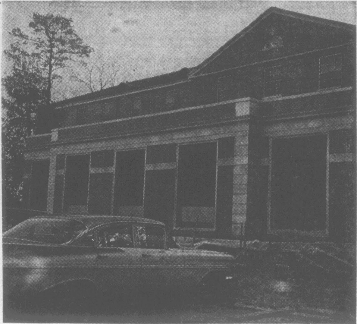
NEW FRONT AND LOBBY . . . for Slay Hall, converted this year to a women's dormitory, is nearing final stages. A lobby and parlors also were added to Umstead Dormitory, also converted this year to a women's hall.
