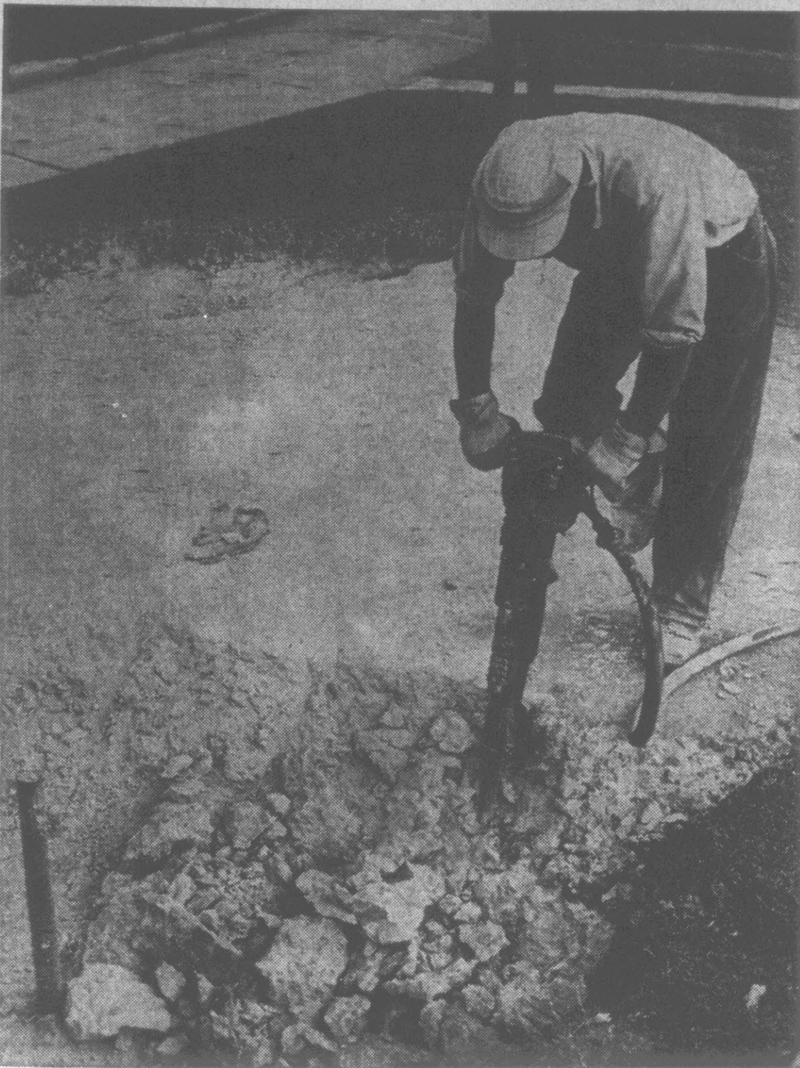
HAMMERING AWAY . . . Worker equipped with air hammer slowly gives huge concrete foundation a "shave."
