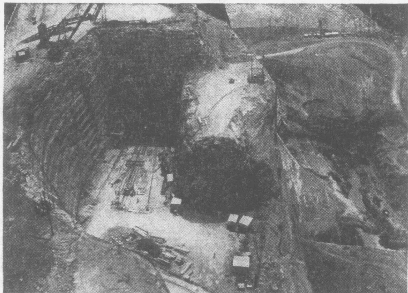
Excavation work goes on at giant left spillway, dwarfing men and shacks far below.
