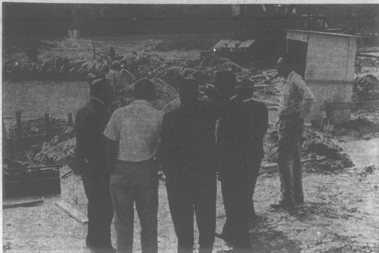
SEWAGE DISPOSAL PLANT CONSTRUCTION SITE . . . Utilities commissioners view progress on the job.
