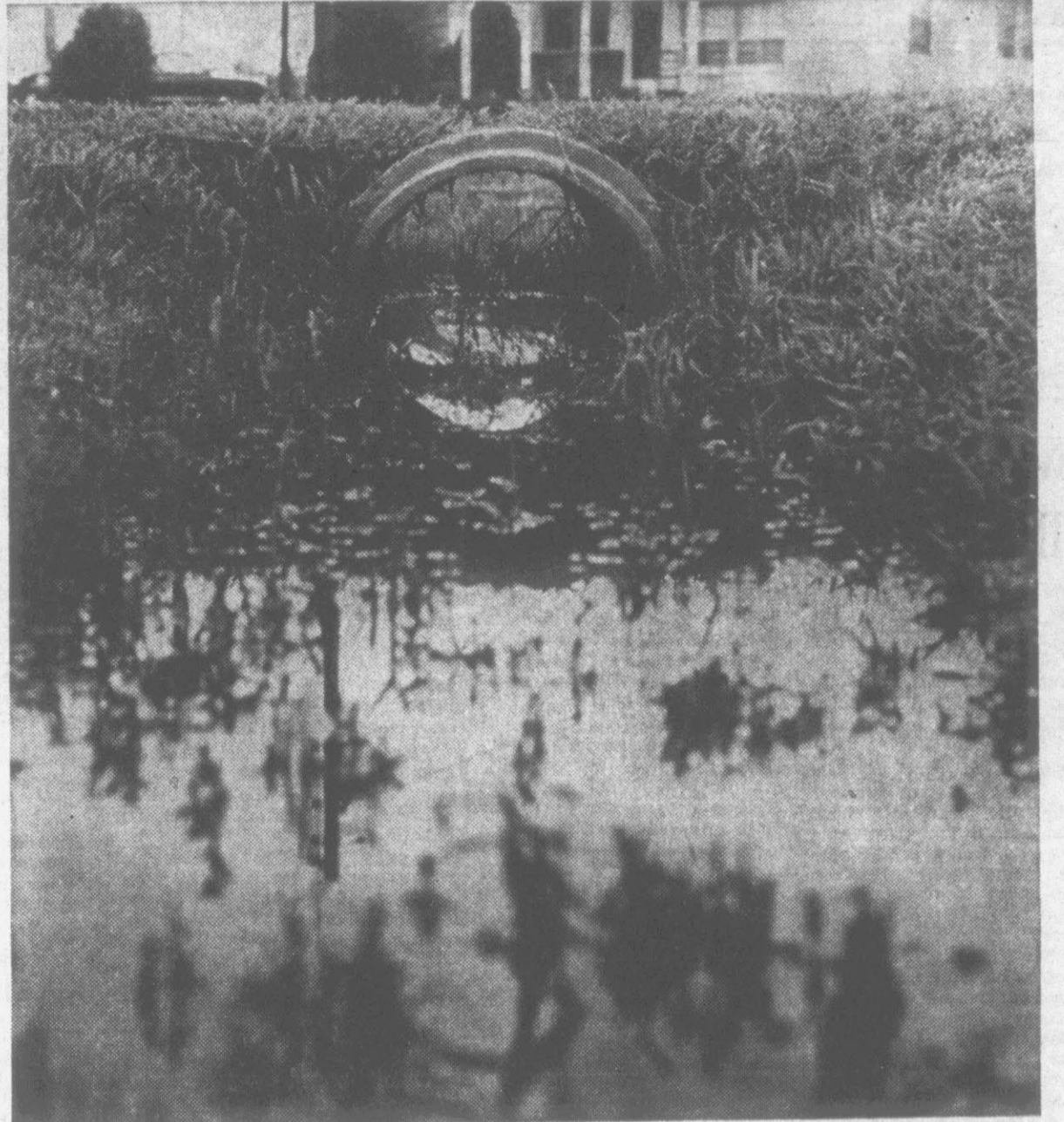
CATCH BASINS WILL HELP THIS . . . flooding is problem on many dirt streets.
