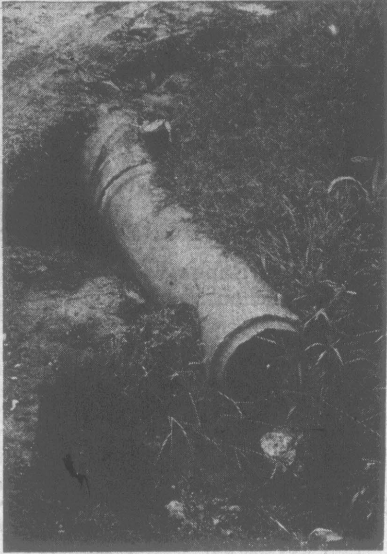
DRAIN PIPE WASHES . . . as rain waters rush off dirt roads.
