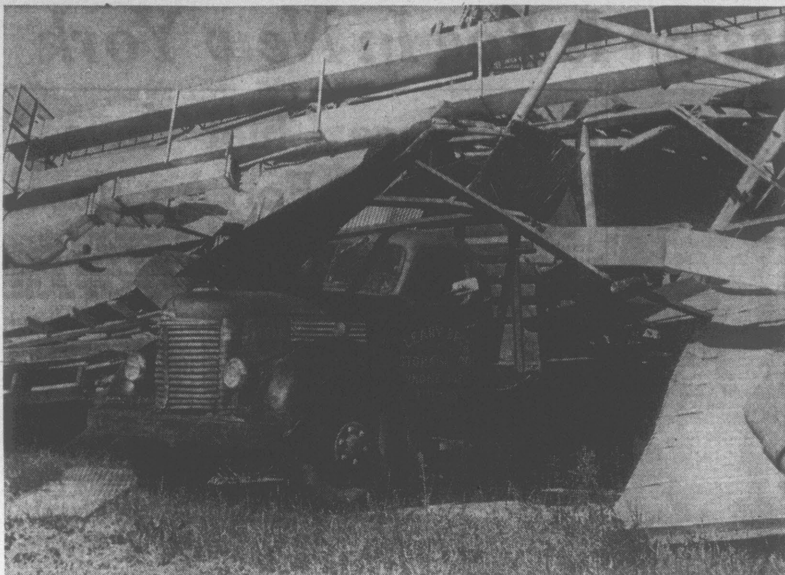
STORAGE BUILDING COLLAPSED—This storage warehouse in Edenton collapsed under the high winds of Hurricane Donna early Monday morning. The supporting metal trusses and sheet metal roofing came crashing down on the truck below. (Photo by Roy Hardee)
