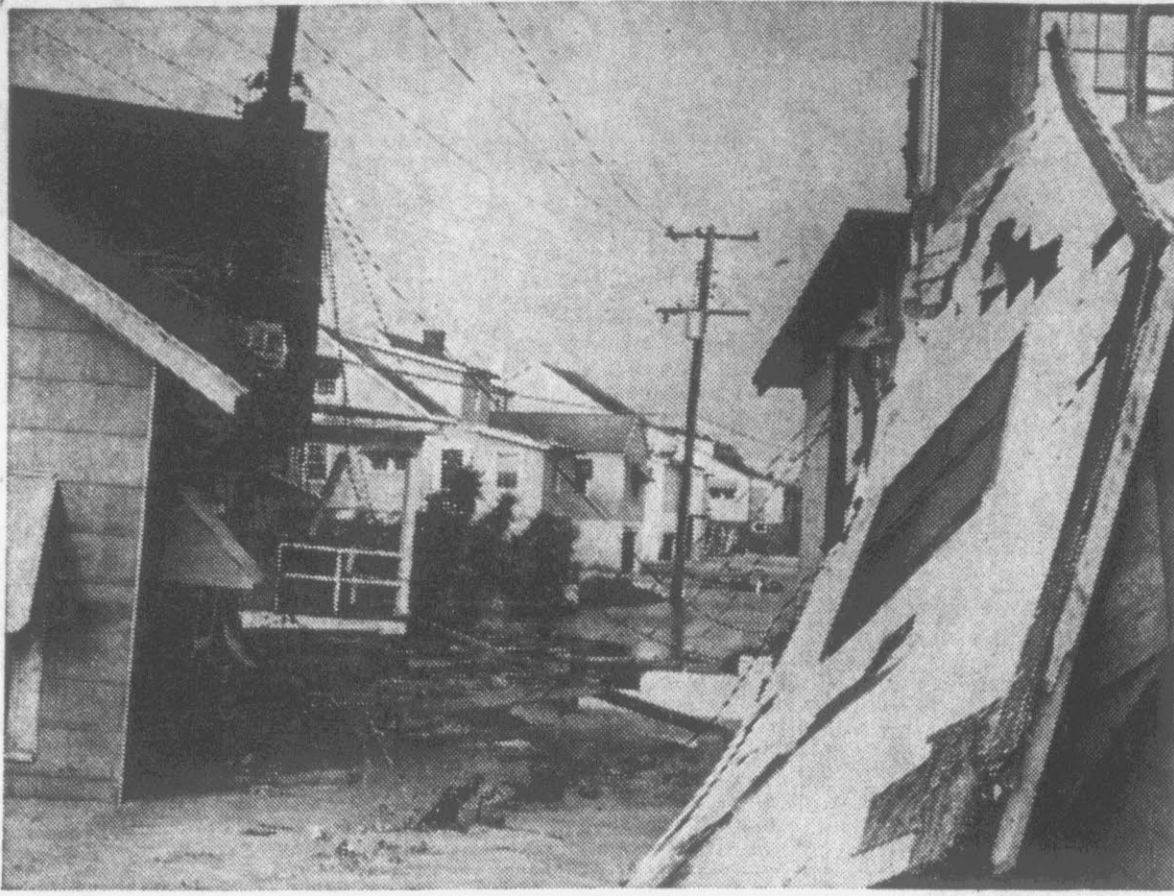
WALL SECTION —leans against its counterpart—the remainder of a beach house—on Atlantic Beach.
