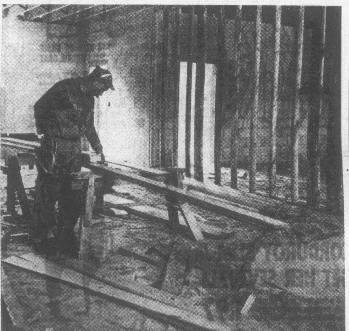
THIS GRIFTON NEGRO SCHOOL . . . will have a lunchroom for serving children when construction is completed. The Pitt County Board of Education says this is part of a program of installing lunchroom facilities for those schools without them.
