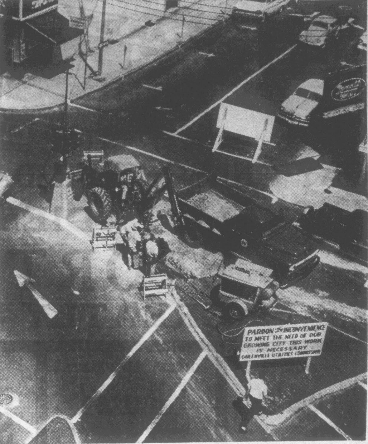
MORE UTILITIES WORK —Reflector Photographer Stuart Savage caught a bird's eye view of Utilities Commission crews as they dug a new electrical manhole at Five Points. The big manhole is part of a long range project to place downtown electrical lines underground. Conduit leading from this manhole will tie in with recently installed lines on Cotanche St. and Evans on the east and to the underground vault at State Bank on the west. Utilities Superintendent Leonard Bloxam said it is anticipated that the manhole will be completed by the end of this week. He said ditches should be filled and the streets patched by Aug. 19.
