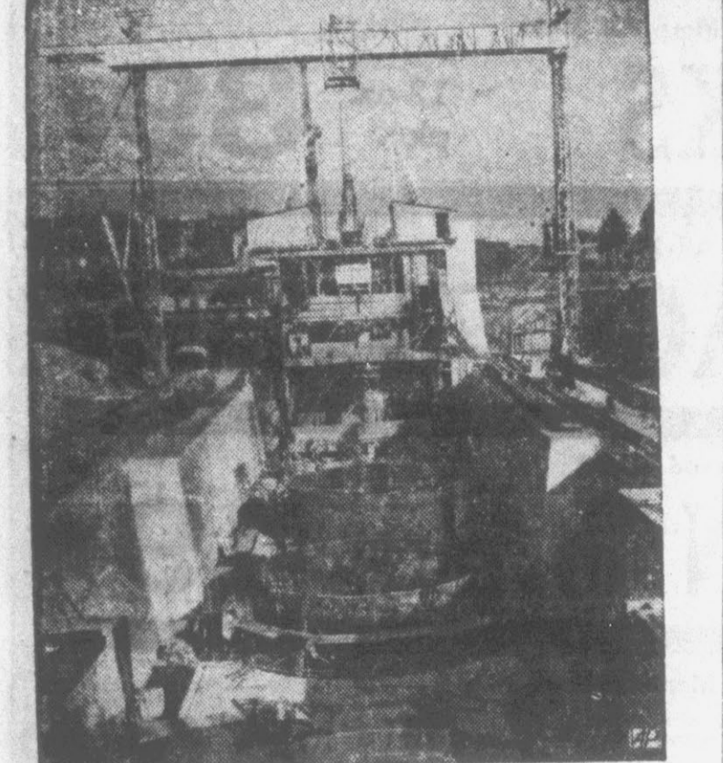
SHIP LIFT—Two huge 180-foot cylinders, capable of hoisting a 1,350-ton ship, are part of the renovation of the Dortmund-Ems canal at Henrichenburg, West Germany.
