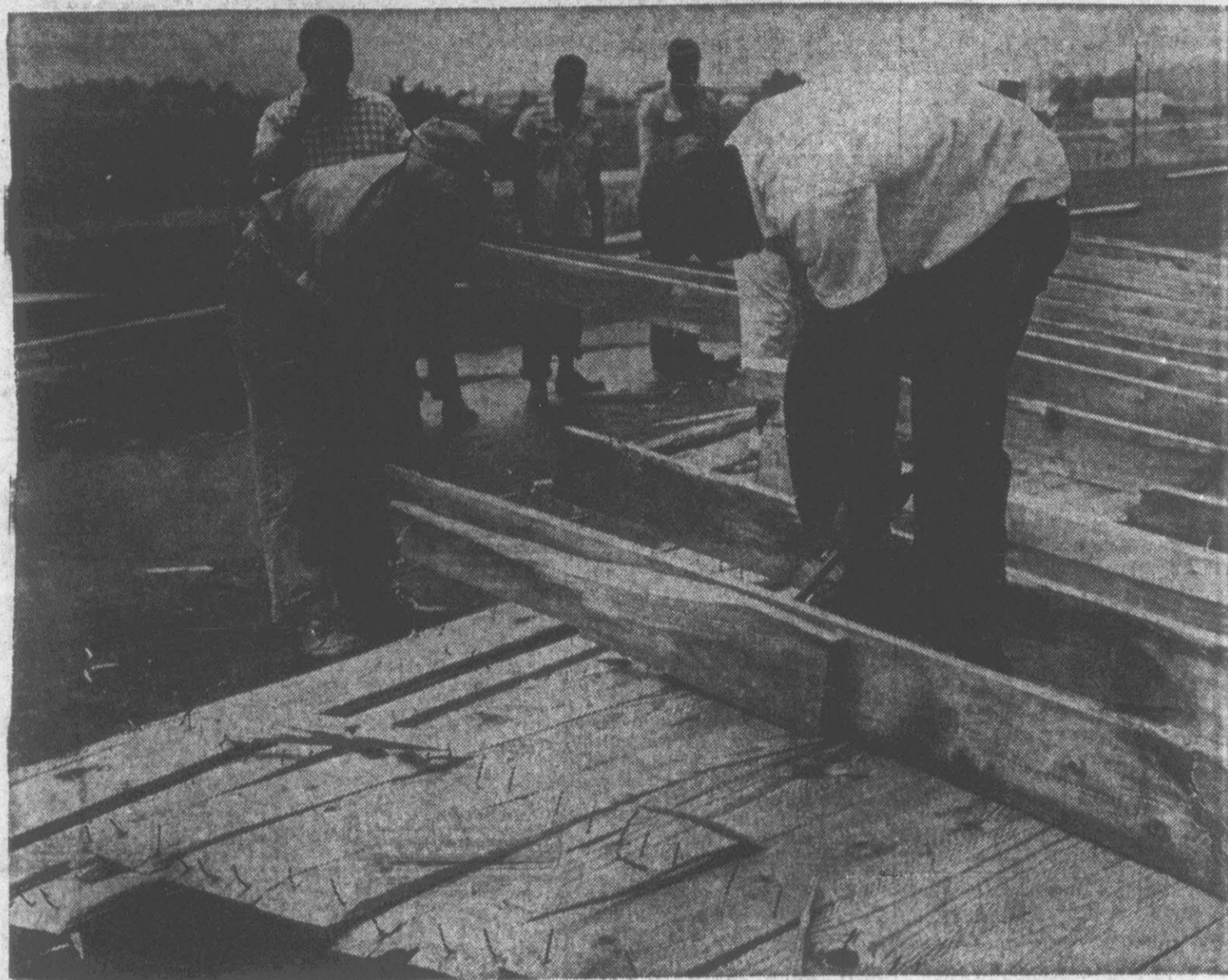
HIGH WINDS . . . resulted in roof damage at the Varina Wholesale Builders Supply in Farmville yesterday. Rain was blown in, causing an estimated $2,500 to $3,000 damage.
