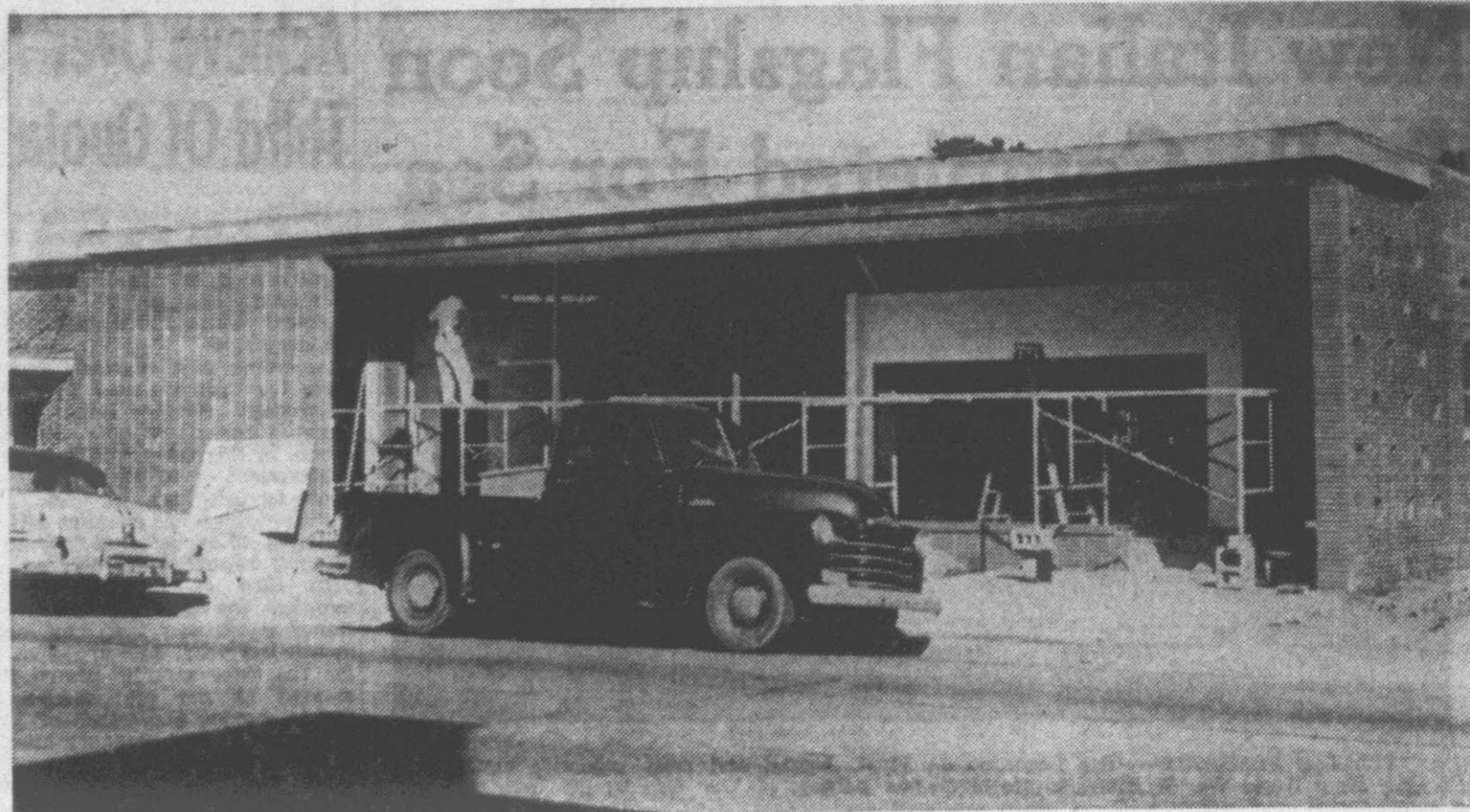
NEARING COMPLETION—Farnville's new post office, situated on N. Main St. between the Williams and Fitzgerald medical clinics, should be ready for occupancy in several weeks, according to construction spokesmen. Farnville finally obtained the new facility after more than a 30-year wait. Dr. Rod Williams is financing the project on a lease basis.
