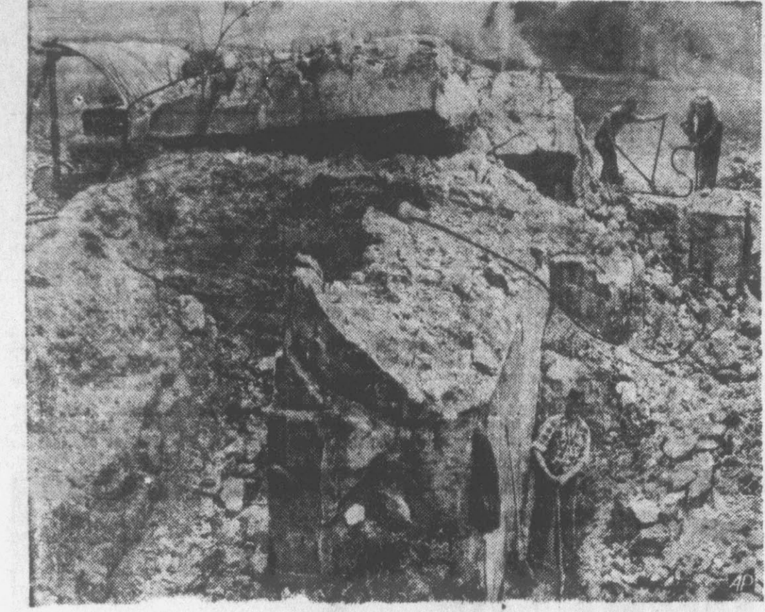
ERASING THE LINE — Workmen start demolition of a portion of Hitler's Siegfried Line at Landau, West Germany. It will take several years for complete eradication of this "West Wall" for hundreds of pillboxes must be levelled in the region.
