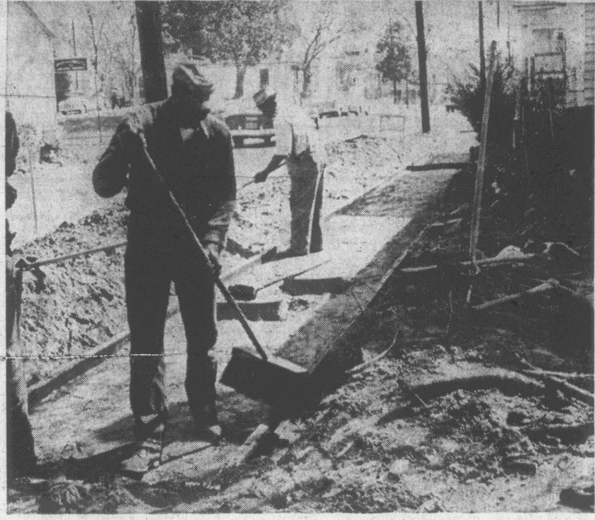
NEW SIDEWALK—A sidewalk is being installed on Second St. between Evans and Cotanche. City Manager Leonard Bloxam said the paved walk will extend the entire length of the block on the south side of the street. Sidewalk will be placed on the north side in front of the Rivers and Associates office property. Bloxam said the walks will be set back to allow for future widening of the block. Cost of the work is being borne by property owners. (Reflector Staff Photo)
