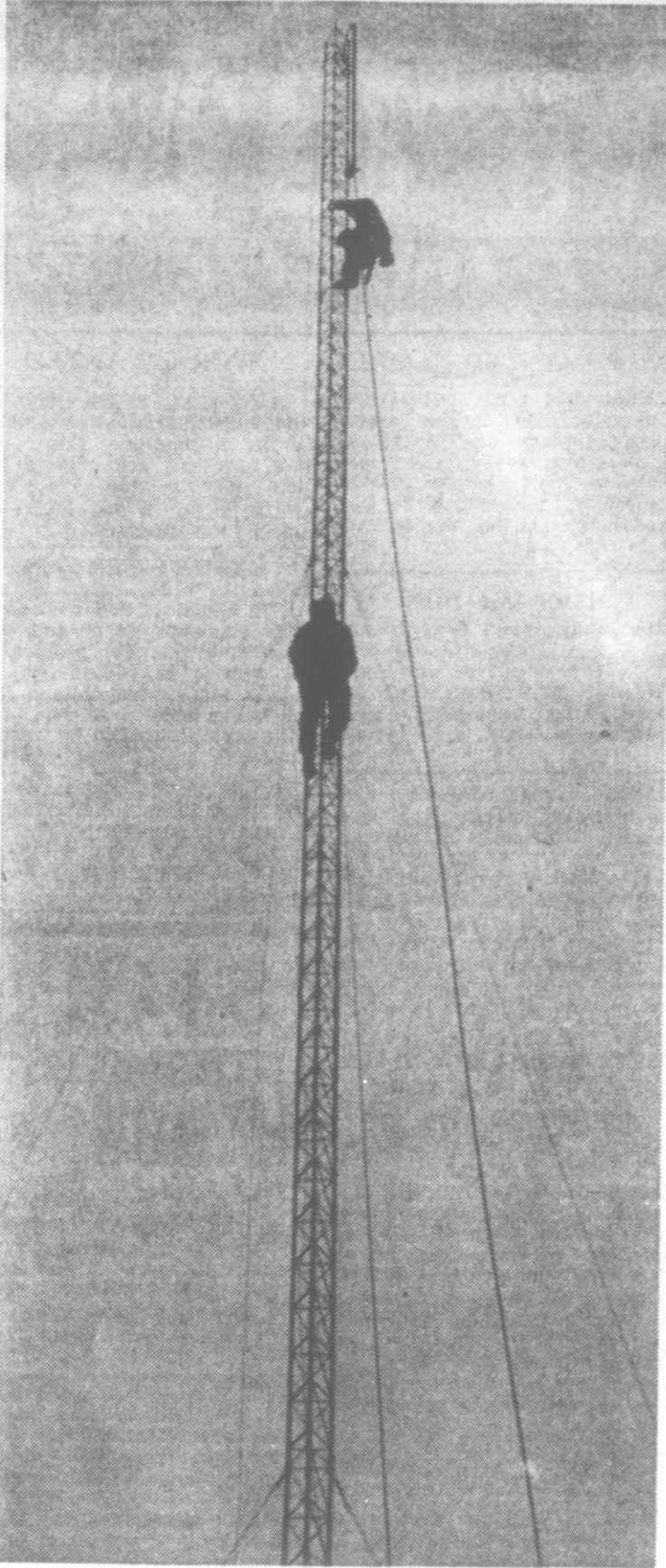
GOING UP IN THE WORLD—These tower construction workers from Gastonia are over 100 feet off the rooftop of Helms Motor Express Inc. on Wilson St. The firm is installing the 150 foot tower as part of their inter-office radio communications system. It took the tower men four hours of work in the cold and wet weather to reach the 110 foot level just above the "top" man.
