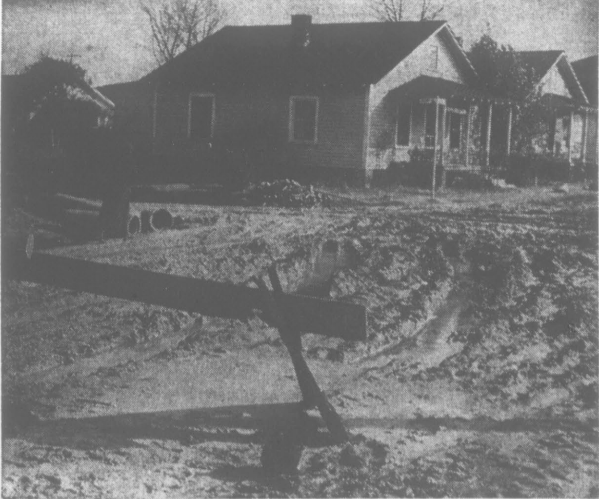
MUDDY STREETS—Vance Street, south of Fifth St., is closed to traffic due to the wet weather and the construction work being done there. City workers have installed storm drainage pipe in the street, which will run from Fifth St. to an open drainage ditch between Fleming and Mack Sts. According to City Manager L. P. Bloxam, work is about 65 per cent complete on the project.
